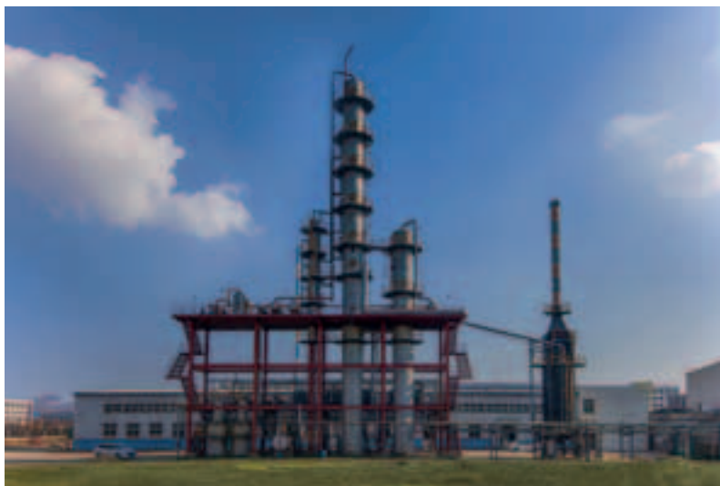
Yantai renewable oil project - Distillation column 煙台再生油項目－蒸餾塔
