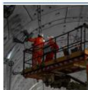
Installation Work Safety Lighting
