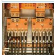
Negative Return Disconnect Panel
