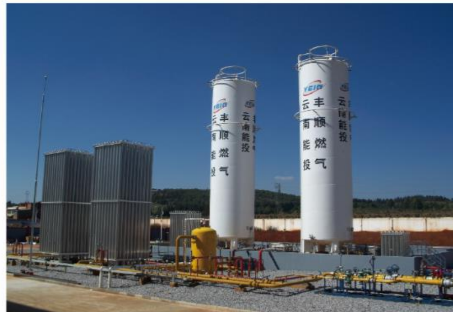
集团宣威丰顺天然气加气站 Fengshun Natural Gas Station of the Group in Xuanwei City
