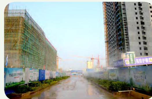
施工现场设置围墙喷淋 Setting up wall spray at the construction site
