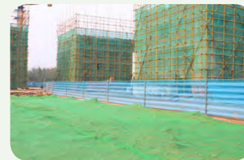
裸露土方进行全面覆盖，设置标准化围挡 Fully covering the bare earth, setting the standard enclosure
