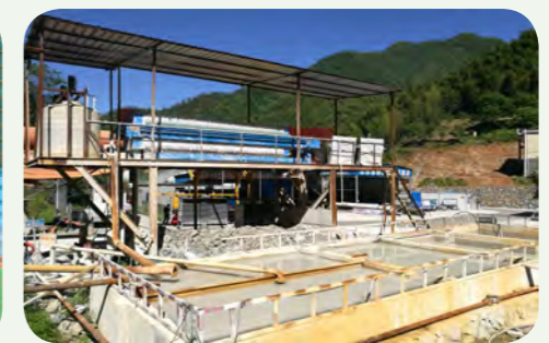
施工现场沉淀池处理拌合废水 Construction site sedimentation tank treatment of mixed wastewater
