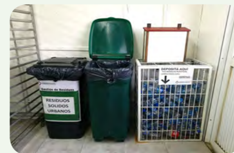
施工现场垃圾分类回收 Waste separation and recycling at the construction site
