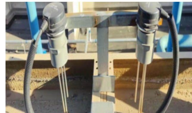
Upgrading make-up water pumps to energy efficient products
