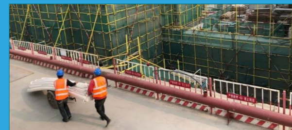
Gradual resumption of work of Jinchen Mansion project in Beijing City Centre
