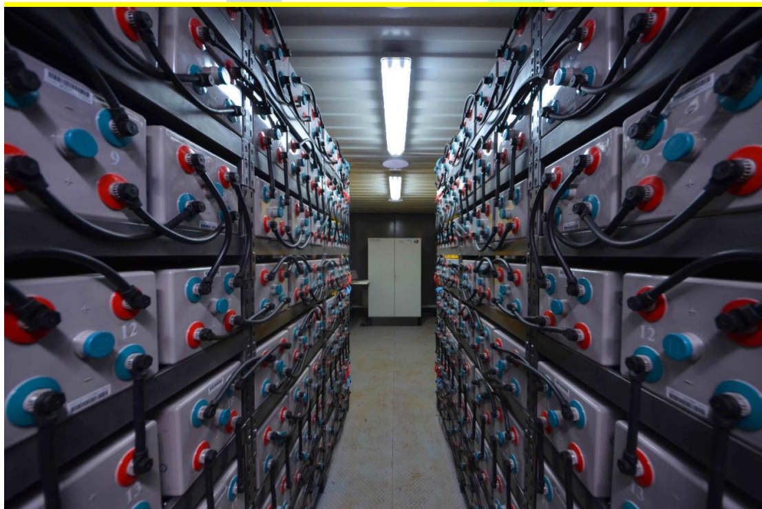
(Valve-Regulated Lead-Acid Batteries In Energy Storage Stations,
