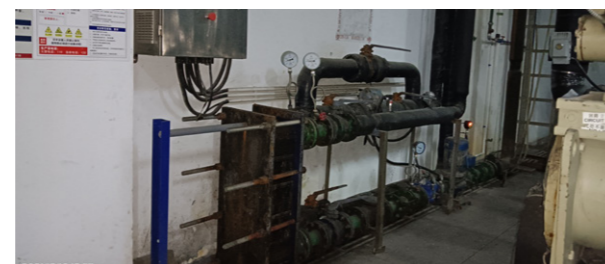
Water circulating cooling system of emulsifying pot
