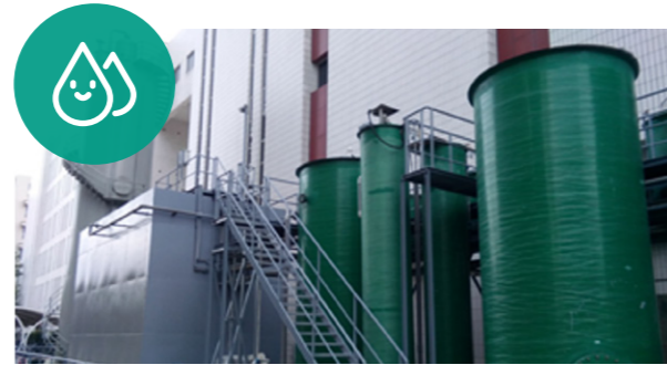
Photo of sewage treatment station of 5C factory
