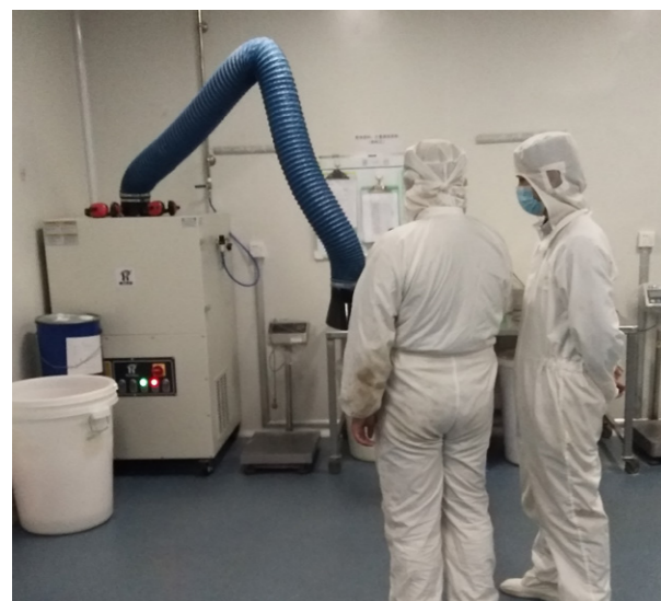
Dust treatment system of the production workshop
