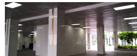
LED energy-saving lighting at outdoor corridors
