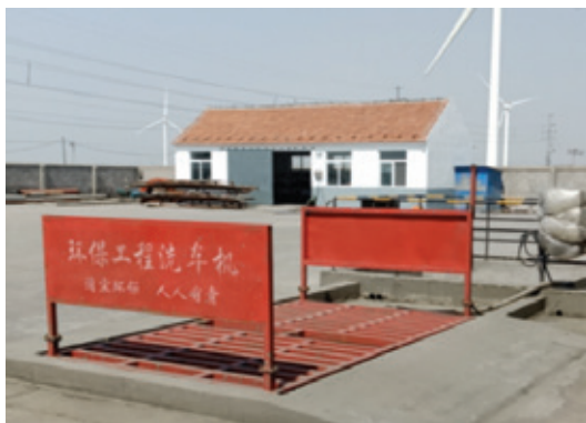
Vehicles washing machine 洗車機
