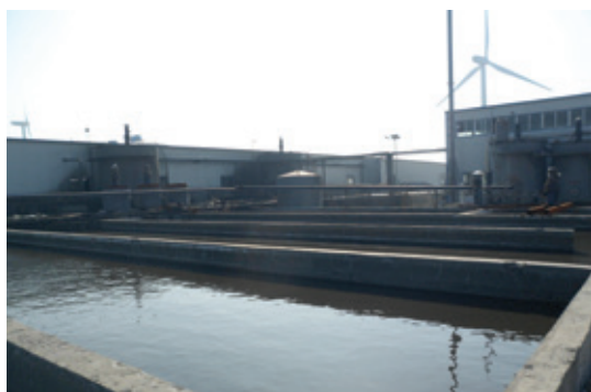
Circulating pool 循環水池
