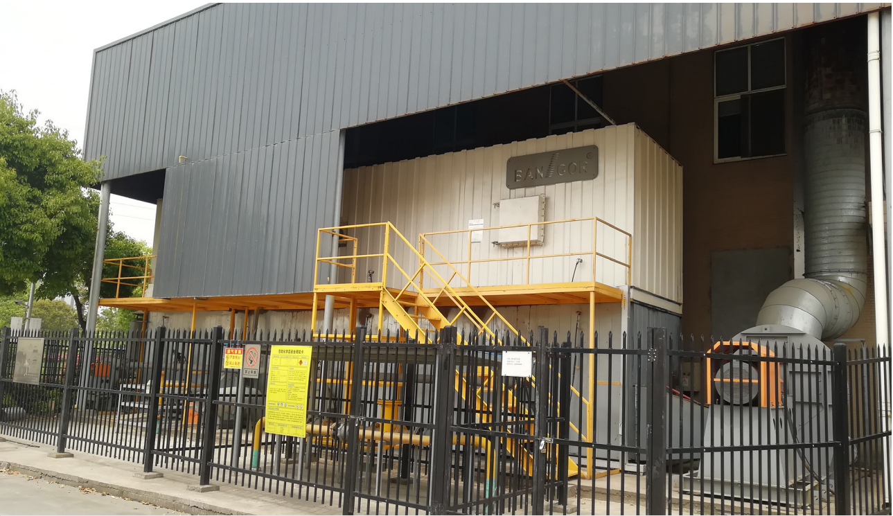
Waste gas treatment facilities
