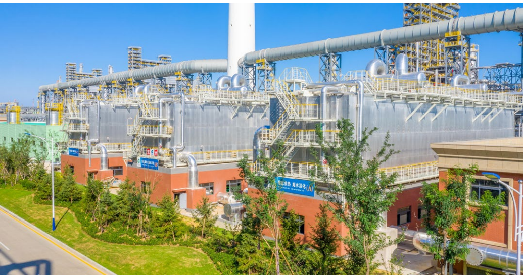
Hengli Petrochemical's seawater desalination facilities
