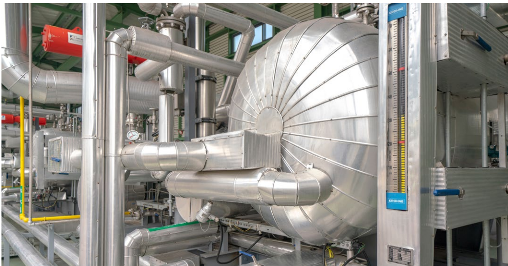
Hengli Petrochemical Refining flare gas transformation
