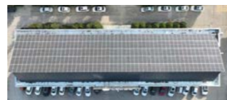
沁水新奥光伏车棚
