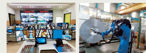
Overhead crane centralized control room Label sticking robot
