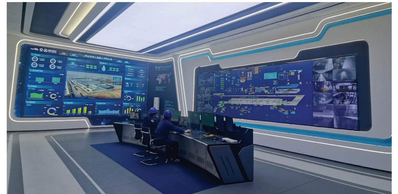
Intelligent Control Center of Taishan Gypsum at Yichang Base
