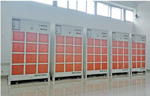
Charging cabinets in the charging areas of operating sites
