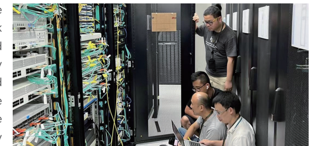
The engineers of the Company are debugging the IT equipment
