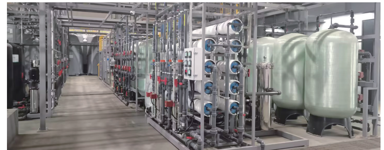
LAZZEN's electroplating wastewater treatment system
