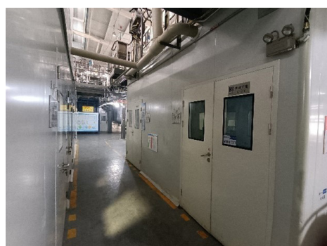
Noise Reduction Project of Refrigeration Machines by Xinxiang Haibin
