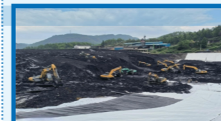
The construction site of the second-phase pollution control project of Hongtai Manganese Slag Repository in Guzhang County
