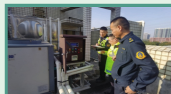
Inspection of key parts
