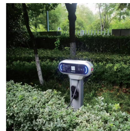
Electric Vehicle Charging Station
