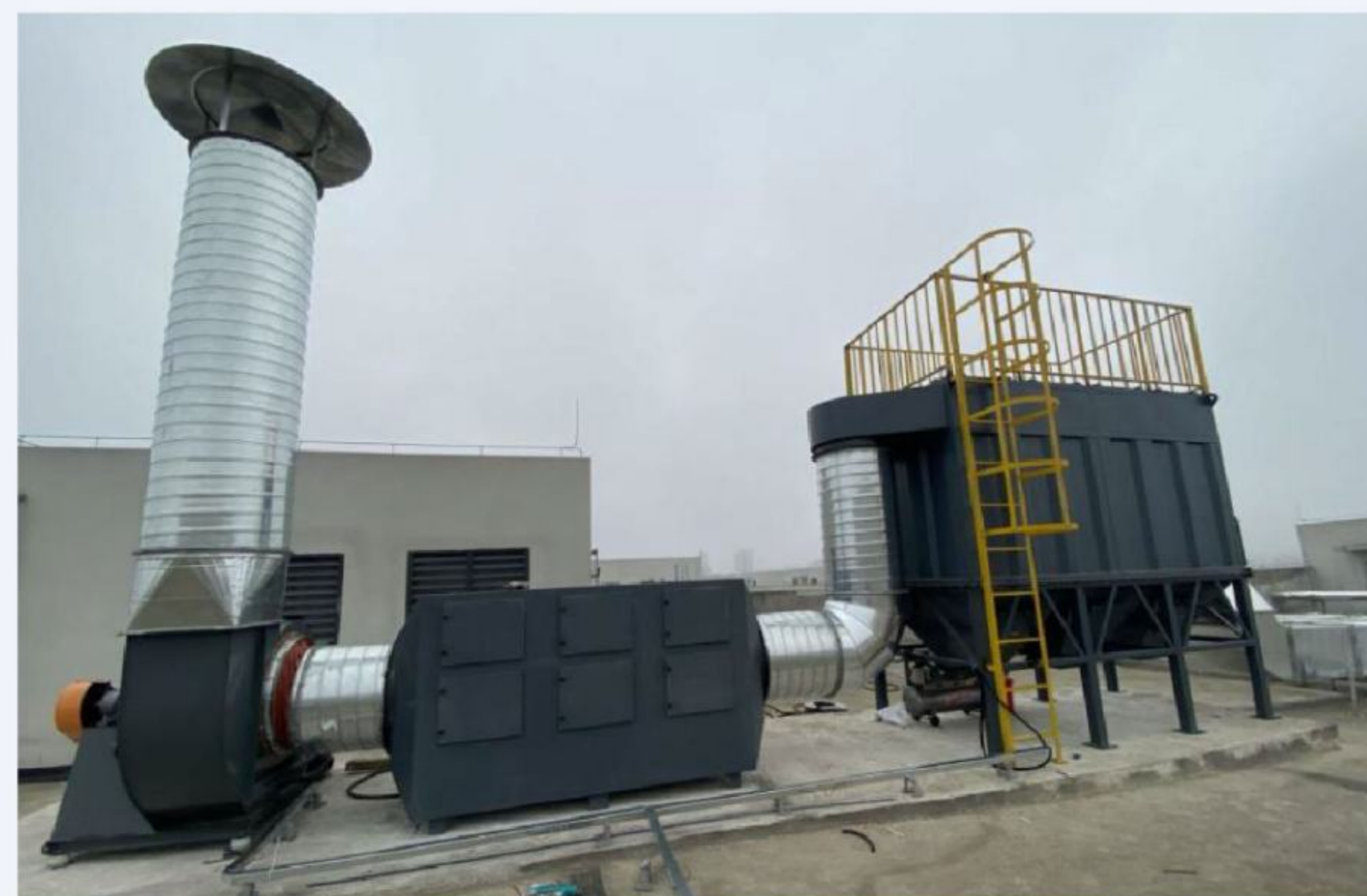
Waste gas purification device
