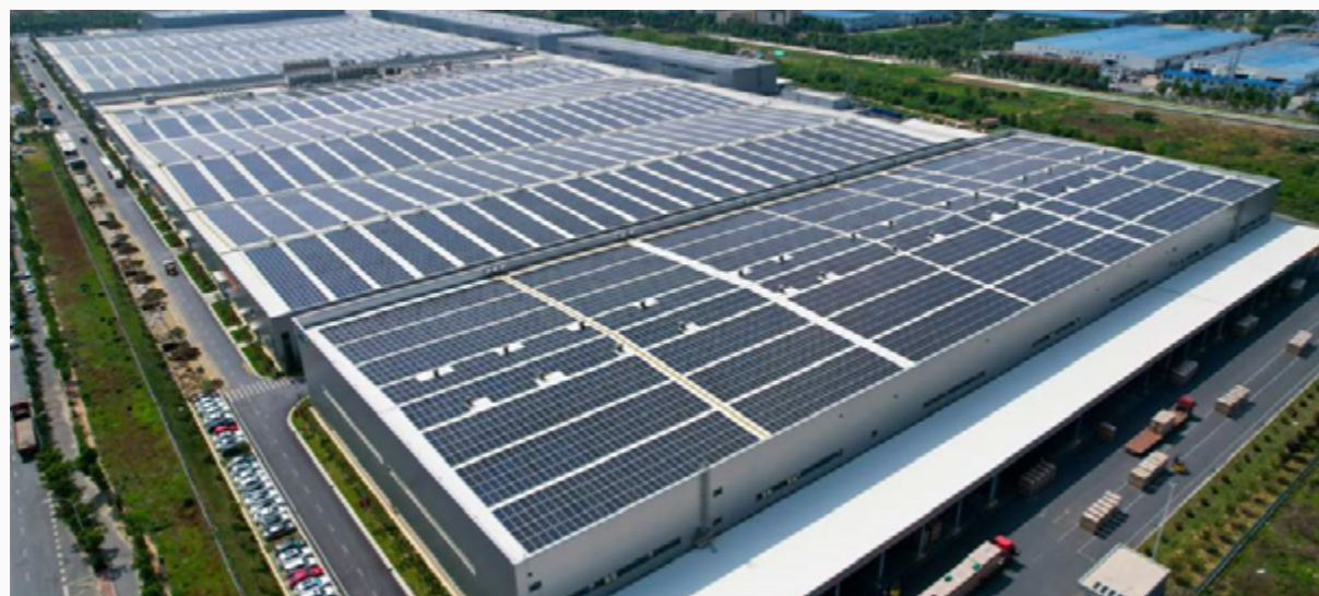
Hefei GCL SI Xinyu PV Power Station
