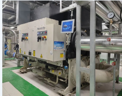
Air conditioning unit in Shenzhen Metro
