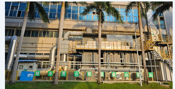
Waste gas treatment equipment
