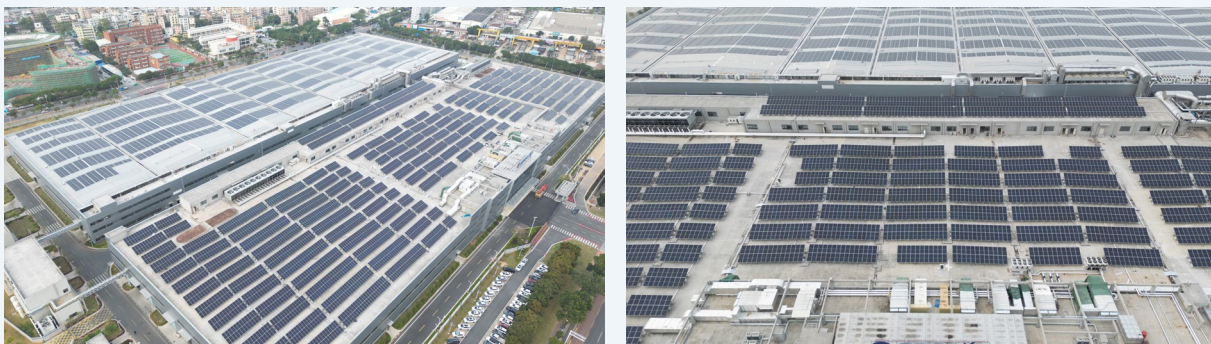
Distributed PV power generation project at Zhuhai Gree Lvkong Technology Co., Ltd.
