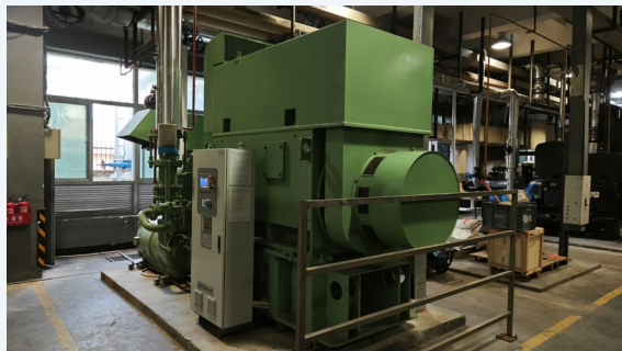
Improving energy efficiency in the air compression station of Zhuhai headquarters
