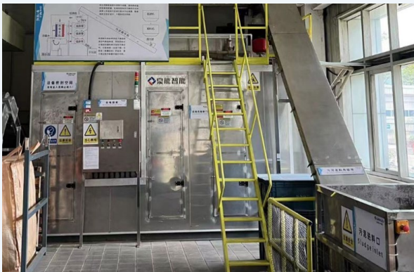
Wastewater treatment equipment
