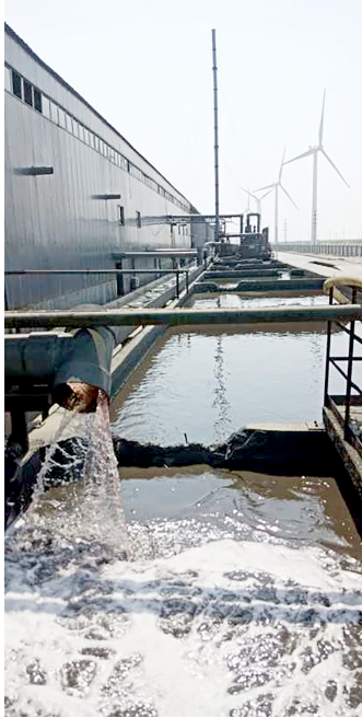
Circulating pool 循環水池
