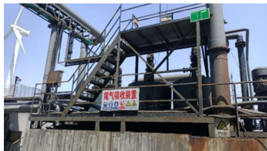
Exhaust gas treatment equipment 尾氣處理設備
