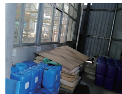
Sewage treatment station before rectification
