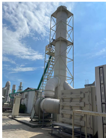
The upgraded organic exhaust gas treatment system
