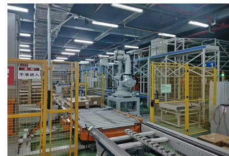
Advanced Production Equipment
