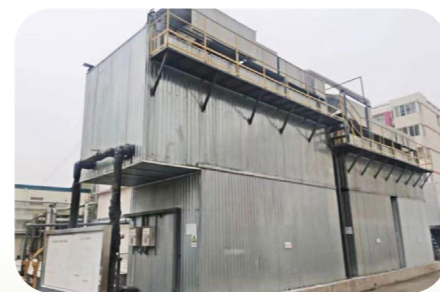
Aima Technology's wastewater treatment system
