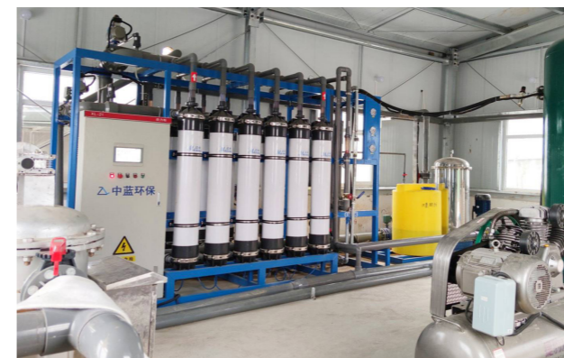
Ultrafiltration Equipment for Water Sources
