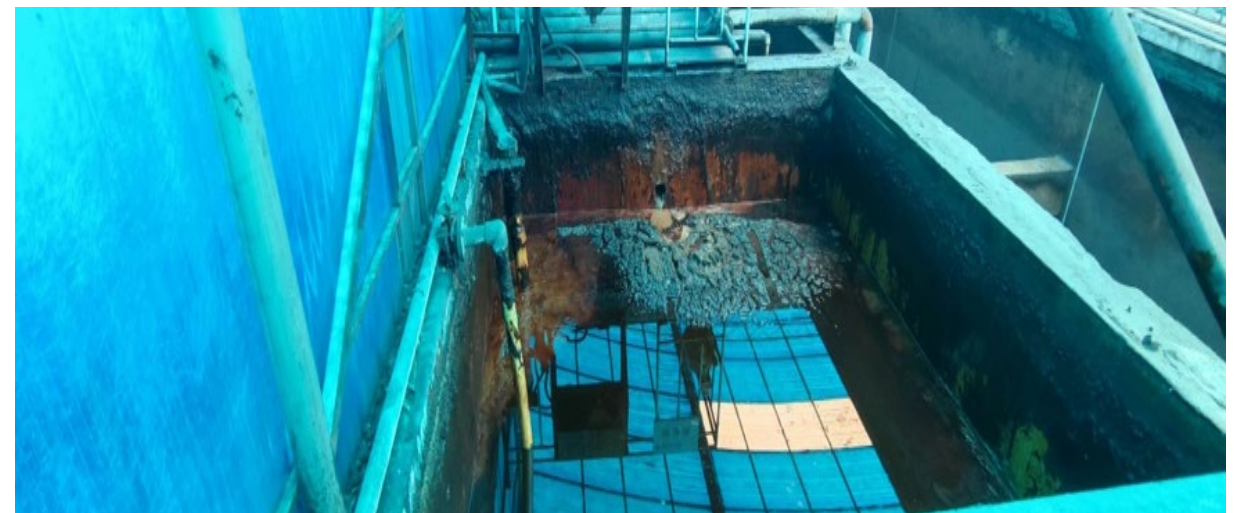
Reduction of Chemicals by the Sewage Treatment Plant of Xiangming Oils
