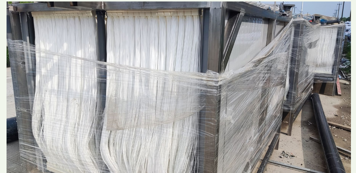
Deep Purification of the "Membrane Bioreactor"
