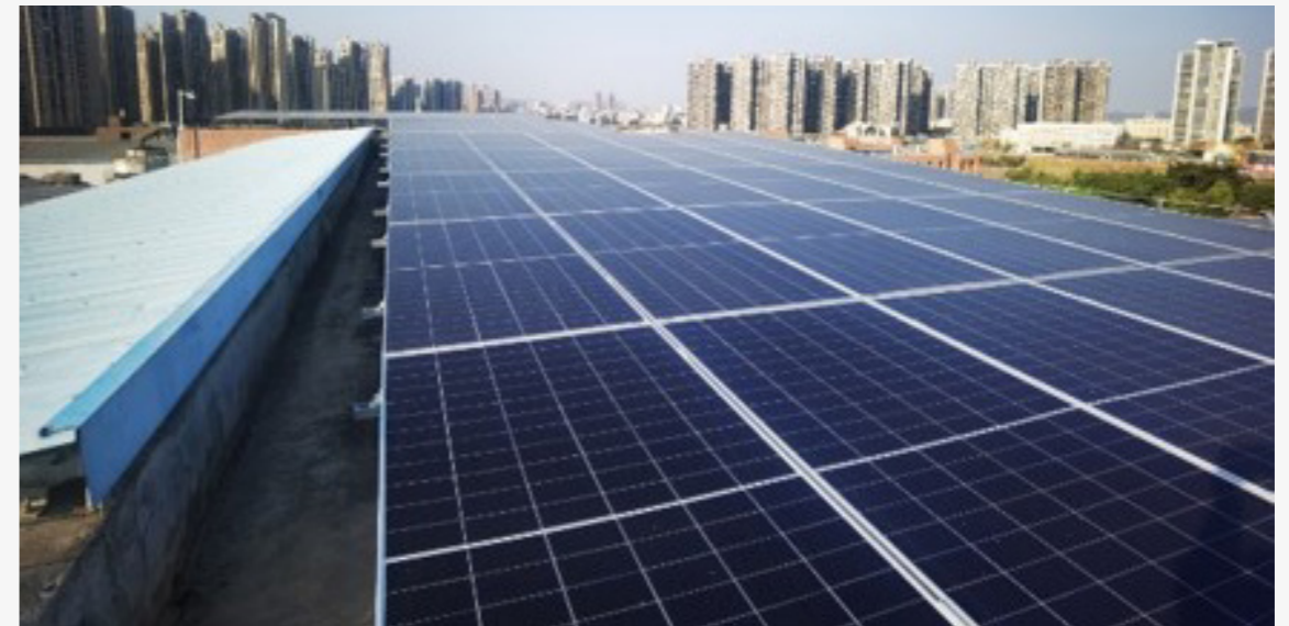
The Huizhou Highpower 0.88 MWp Photovoltaic Project was Successfully Completed and Commissioned in November 2025, Contributing to the Optimization of the Energy Structure
