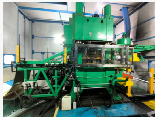
Replacement of the old D7 steam line with the new D7 steam line on Line 8
