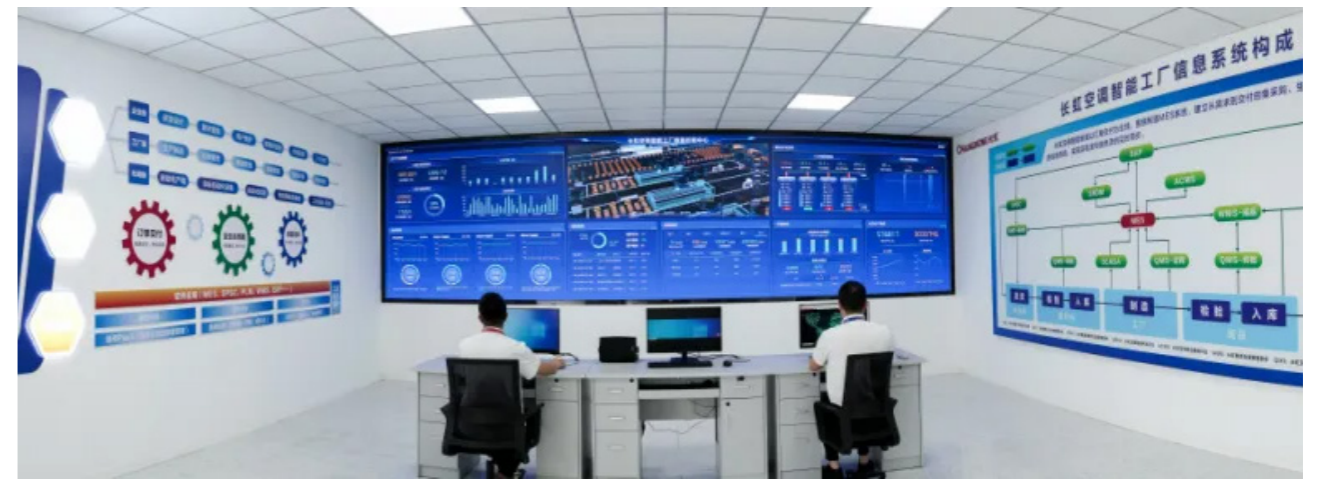
Changhong Air Conditioner Intelligent Control Center
