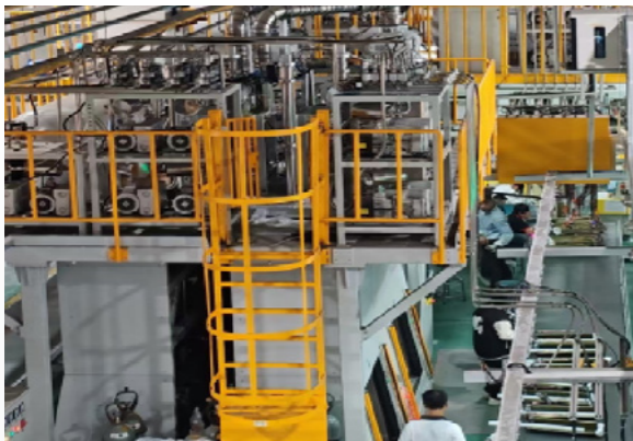
Helium Inspection Line 1 (internal)
