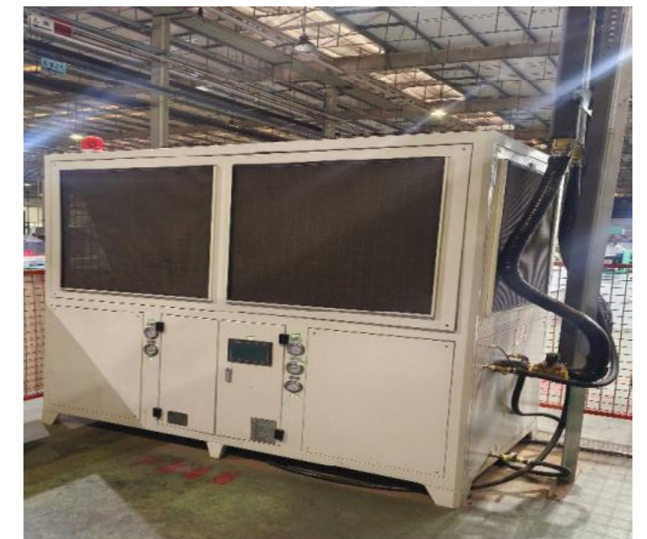
The Company's manufacturing plants commissioned air-source mold temperature units to replace traditional models, achieving electricity savings
