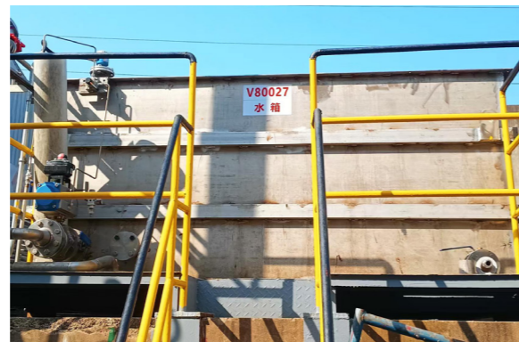
Steam Condensate Recovery Facility
