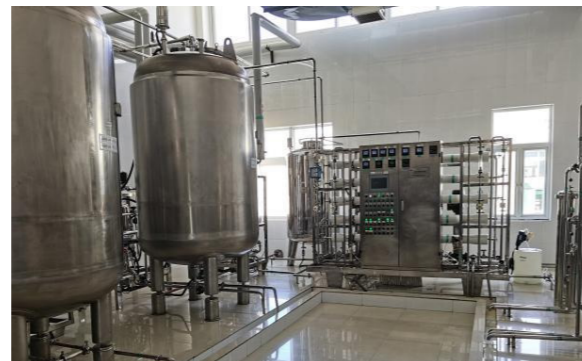
Purified Water System
