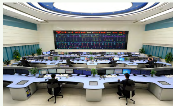
● 集控中心全面部署 Centralized Control Center Full Deployment
