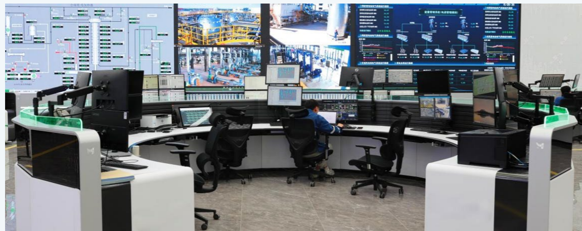
绿色氢基能源（绿电-氢-氨）柔性管控系统 Flexible Control System for Green Hydrogen-Based Energy (Green Power-Hydrogen-Ammonia)
