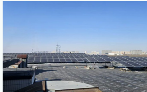
Photovoltaic panels at the Second Chinese Medicine Factory
