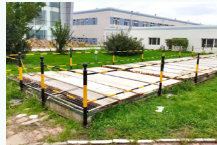
Wastewater treatment station
