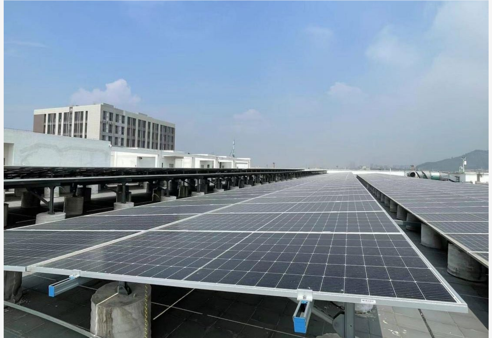
Photovoltaic System at Keerun Warehouse
