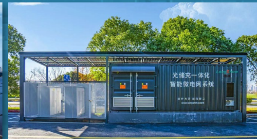
1 MW of Energy Storage Capacity
