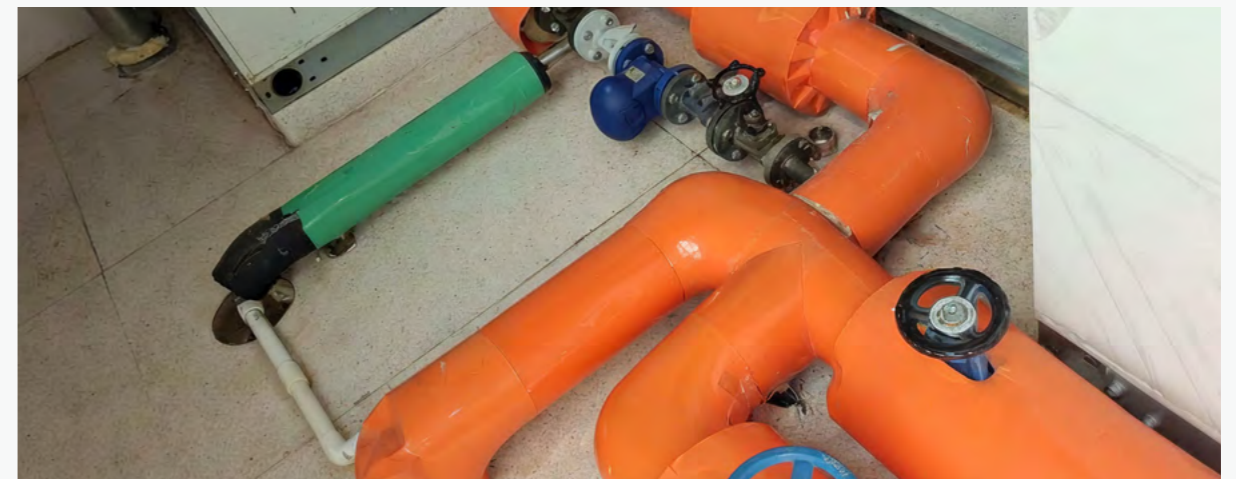
厂区蒸汽疏水阀
