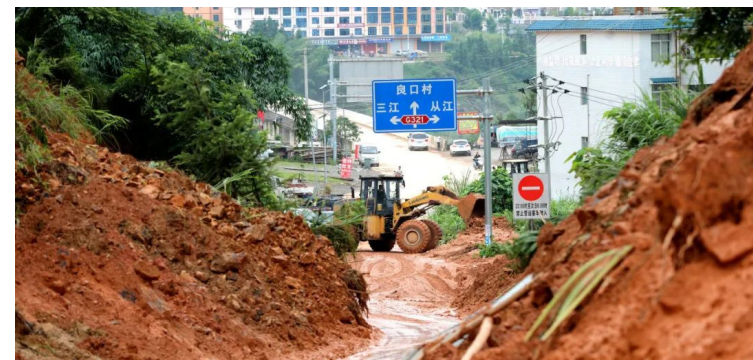
Flood Control and Disaster Relief at Frontline in Liuzhou, Guangxi
