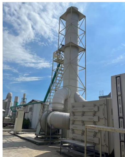
The upgraded organic exhaust gas treatment system
