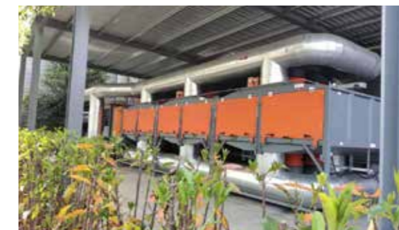
Exhaust Gas Treatment Facilities
