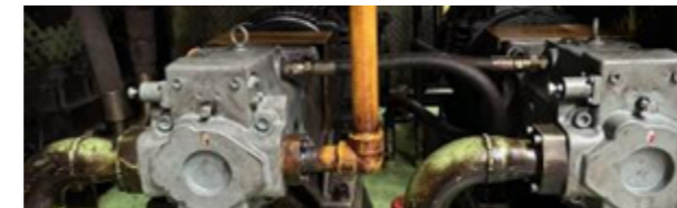
Hydraulic Station Motor Transformation
