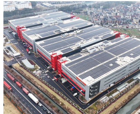
Dahua Smart IoT Industrial Park Rooftop Photovoltaic Project
