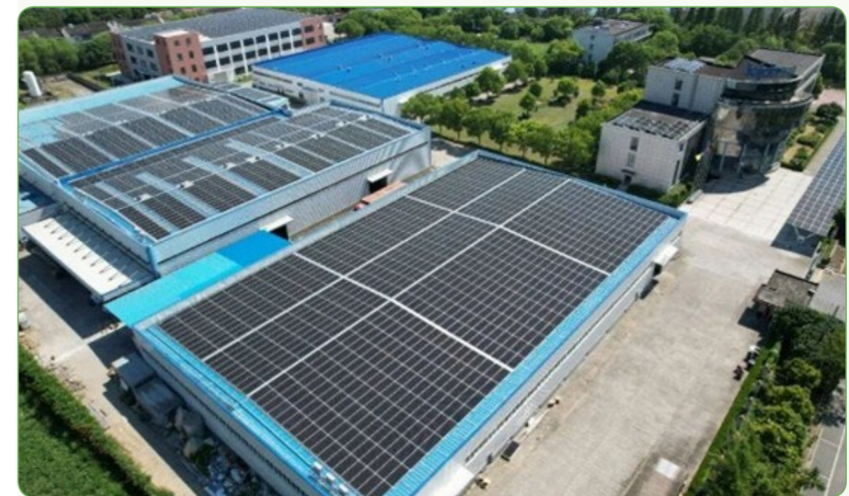
C&D Automobile Phase II 2.2 MW Distributed Photovoltaic Project
