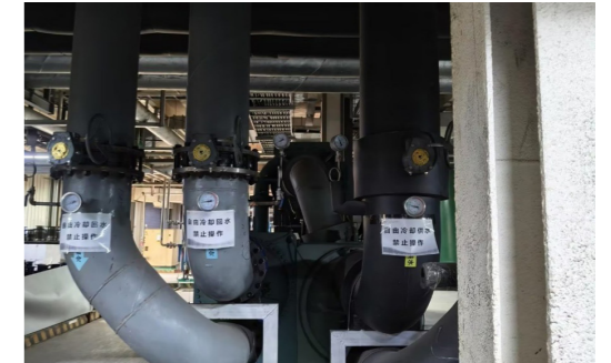
Cooling Water Circulation System of Air Conditioning Cooling Towers of Hongyuan New Material (Baotou)
