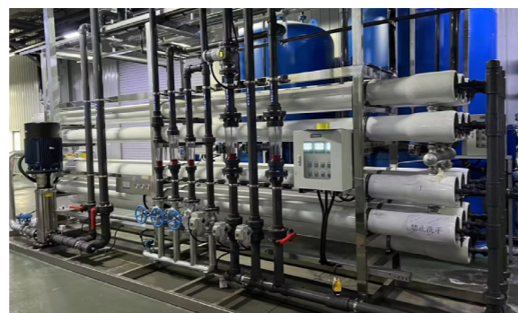
RO Concentrated Water Recovery System of Hongyuan New Material (Baotou)
