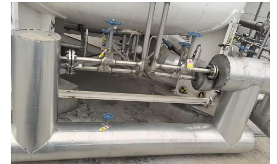
Liquid Nitrogen Recovery and Collection System of Hongyuan New Material (Xuzhou)
