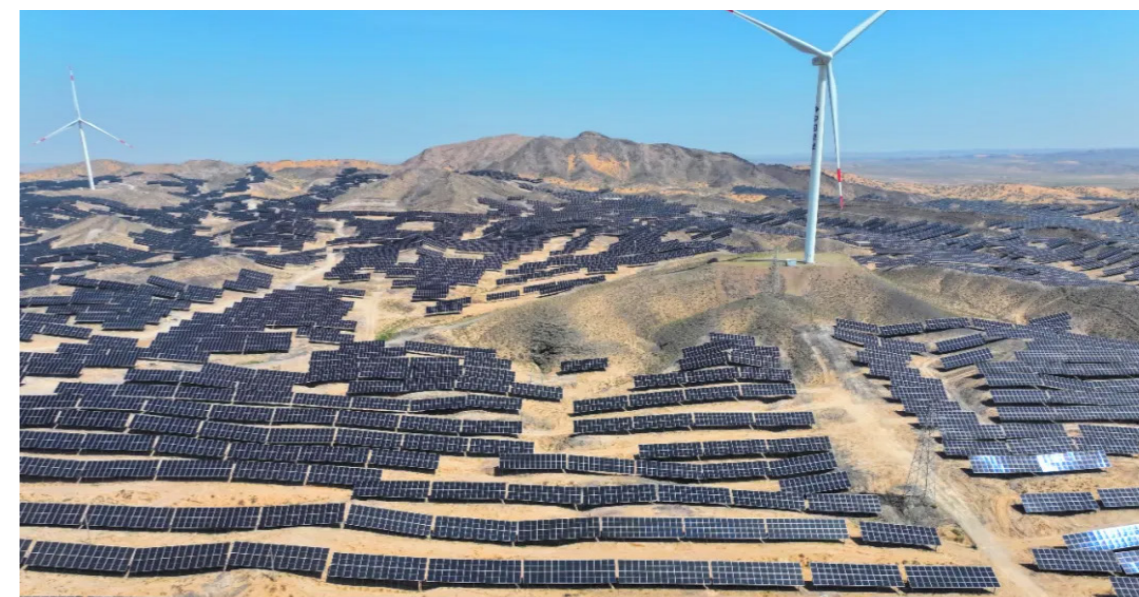
HY Solar Zhongwei Project, Ningxia
