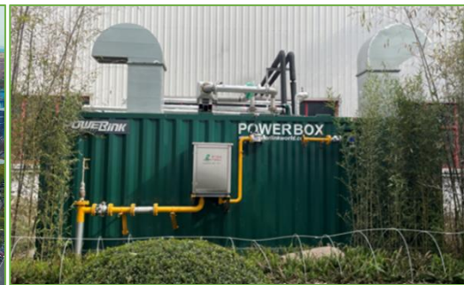
Figure: Tri-generation Unit Project
