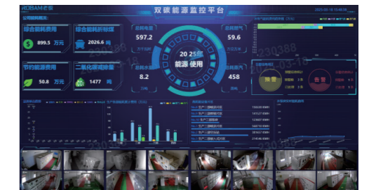
Energy Consumption Management Platform
