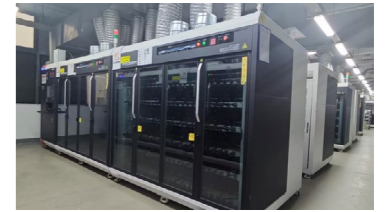
Energy-Saving Aging Room
