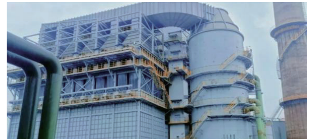
Flue gas desulfurization and denitrification retrofit of the 360 m 2 sinter machine
