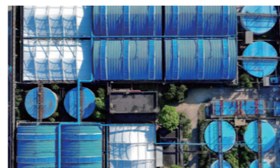
Tail gas collection project for phenol- and cyanide-containing wastewater
