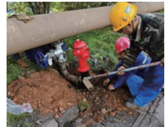
Renovation of the fire water system for the main water pipe supplying the ironmaking plant
