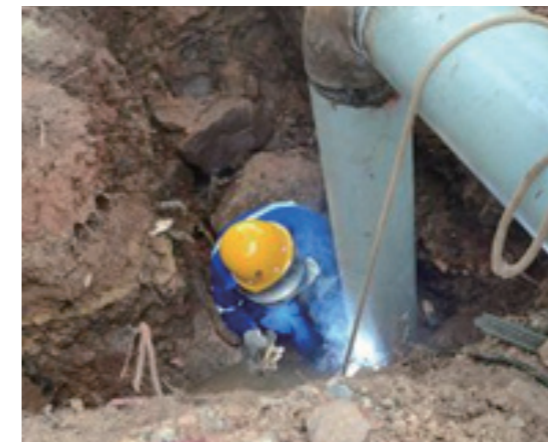
Connection works for the renovation of the main inlet water pipe for the southern pressurized system
