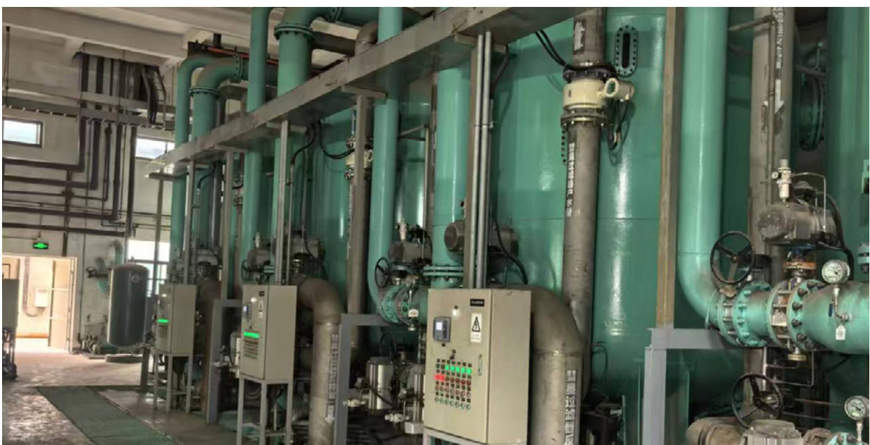
▲ Reclaimed water treatment equipment
