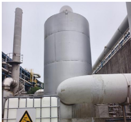
▲ Sodium hypochlorite spray equipment
