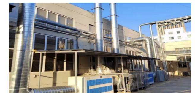
Organic Waste Gas Treatment Facility
